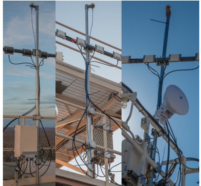
Velocite testing: 4G/5G base station site installation
